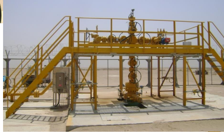
GD and H2S Monitoring
