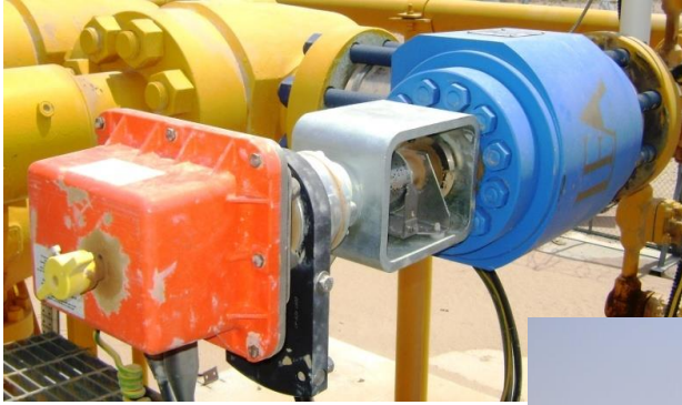
Choke Valve controls
