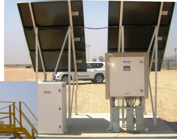
RTU and power supply distribution
